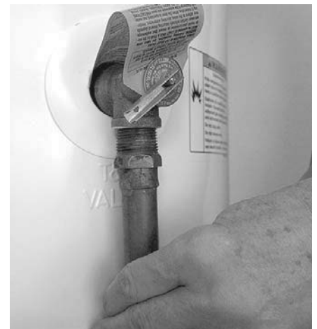
Figure 16 - The T&P Relief Valve discharge pipe must be installed properly and piped to an adequate drain.
