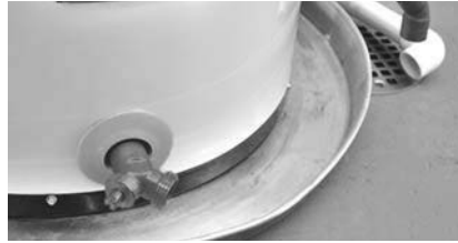
Figure 8 - A suitable drain pan piped to an adequate drain can help protect flooring from leaks and drips.
